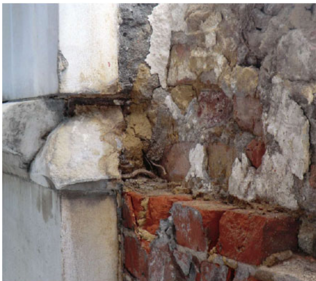
Image showing the poor quality brickwork behind the outer skin of stone.
