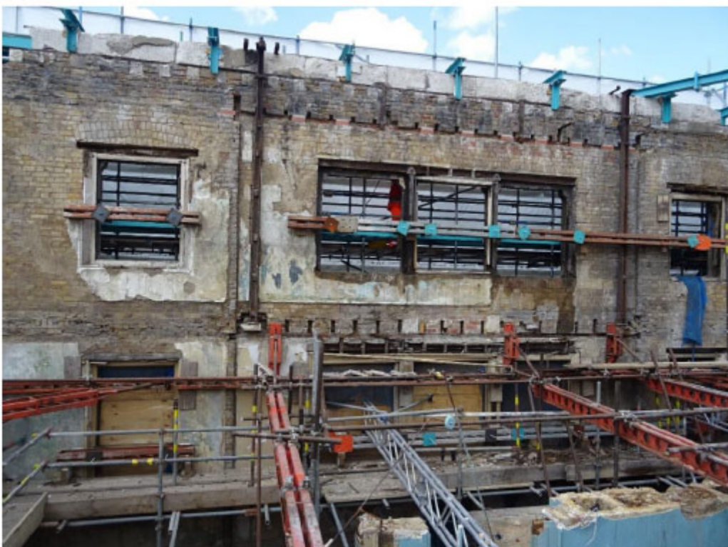
Image showing rear face with decaying brickwork, rotting timber and corroded metalwork.
